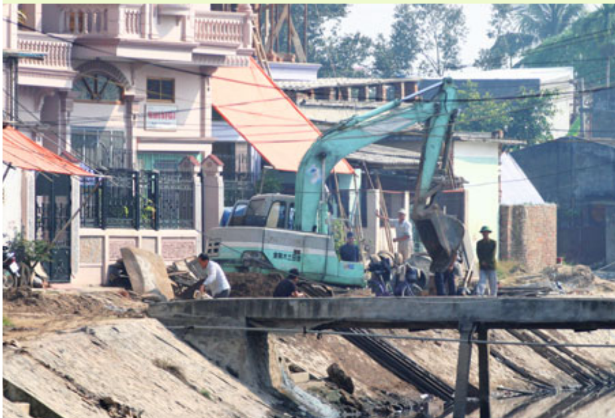
The open sewer network in the city of Haiphong was repaired and the beaches cleaned. Photo: Jari Tenhunen
